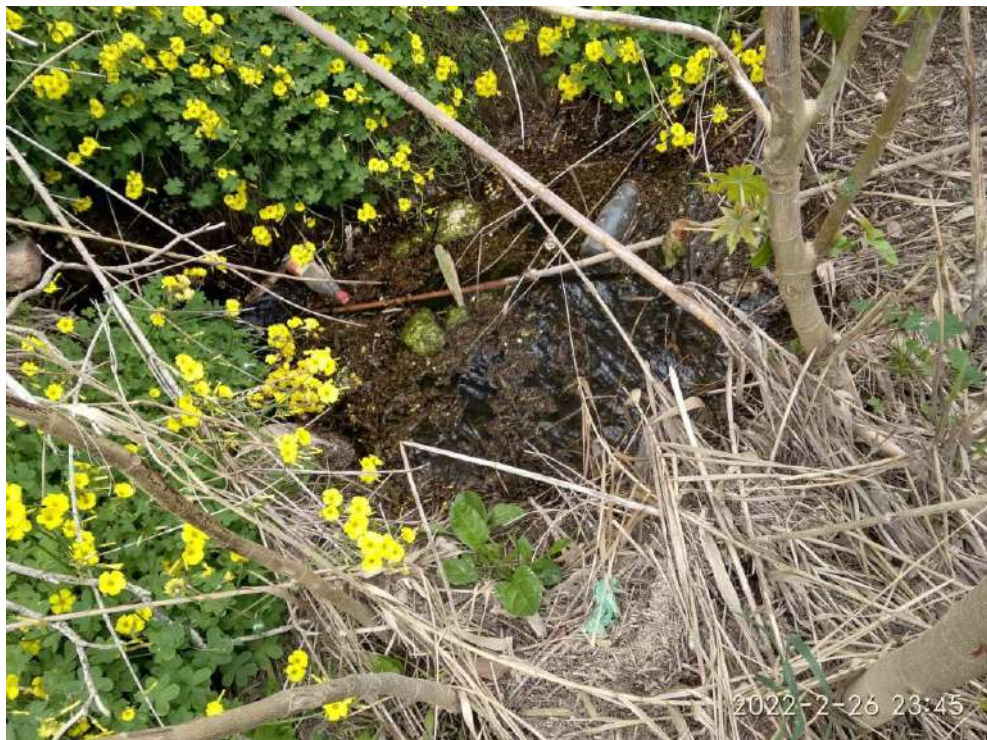
FIGURE 66: POND WITH WATER AT THE DISCHARGE POINT OF THE BURIED PIPELINE CROSSING THE ROAD LEADING TO THE DELIMARA POWER STATION
