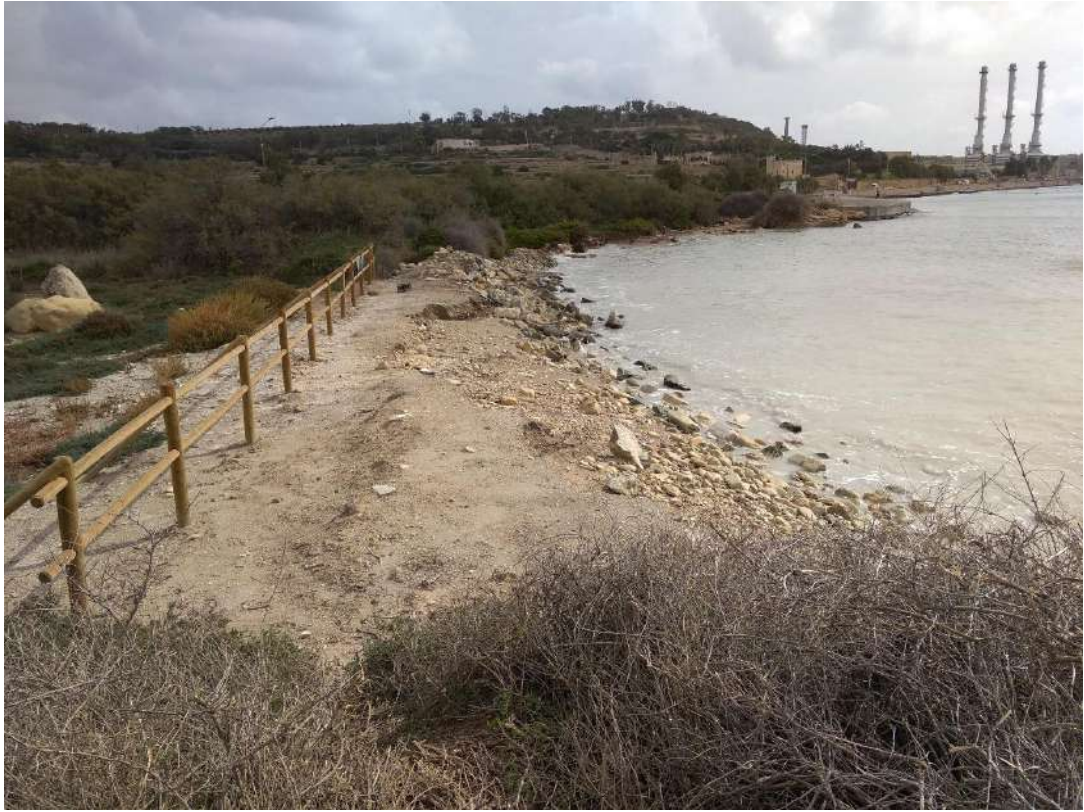
FIGURE 47: STATUS OF COASTAL EROSION AS NOTED ON 27 TH OCTOBER, 2021
